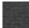
B5 - Dark grey brick Location: 'Tower' block / 'Shoulder' block - projecting stretcher bond detail
